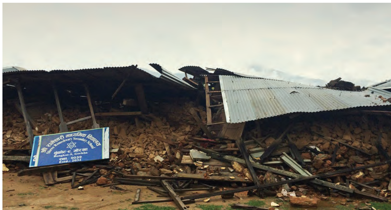
A school in Gorkha completely destroyed by the April 25th earthquake.
