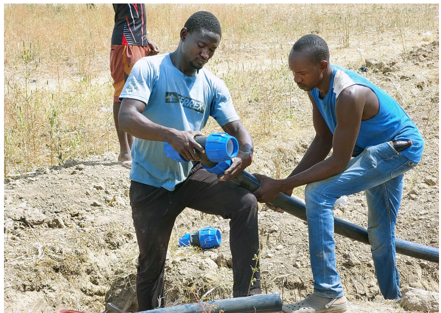
Workers construct a household water connection for a family in Ghana's Builsa AP.
