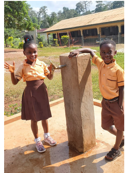
Above, schoolchildren show off their new school water tap, provided by World Vision. “World Vision has helped us to address our water and sanitation challenges in the school,” says Kingsley, the head teacher at Anglican Basic School.
